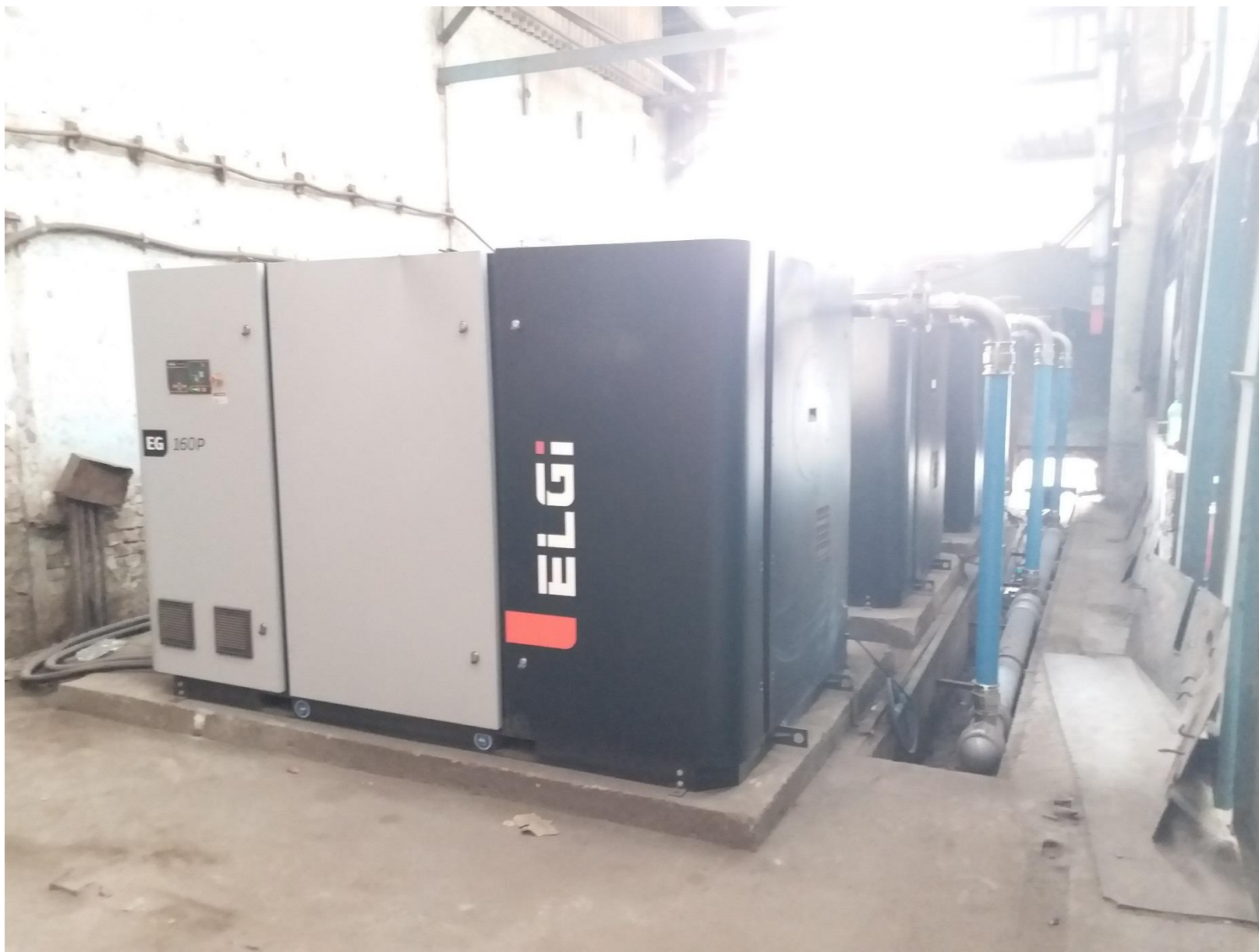
Compressors with interconnecting Transair Pipeline
